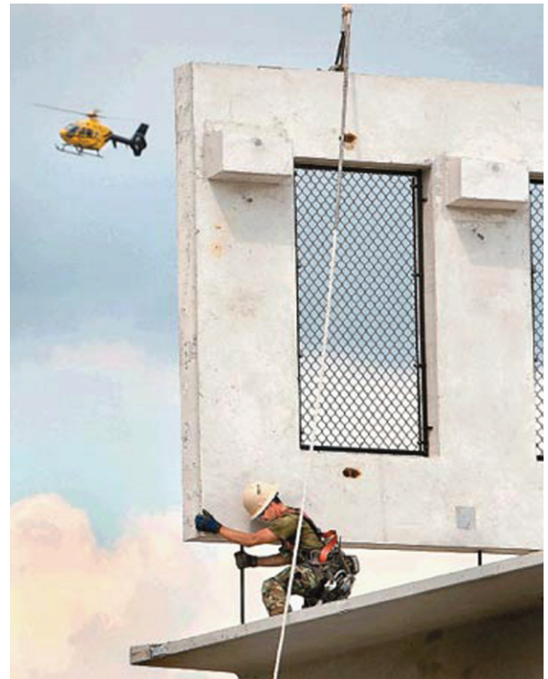
Sam Abrell of Winchester, an employee with Shockey Precast Group, aligns a wall section as a crane lowers the building component into place. Abrell is part of the crew building a new parking garage on the campus of Winchester Medical Center, part of an extensive expansion project planned by Valley Health. In the distance, a medical helicopter flies by the work site. (Photo by Jeff Taylor)
