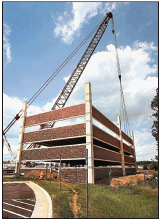
The first phase of the hospital's expansion project — the 560-space parking garage on the east edge of WMC's campus — will probably be complete by November. (Photo by Jeff Taylor)
